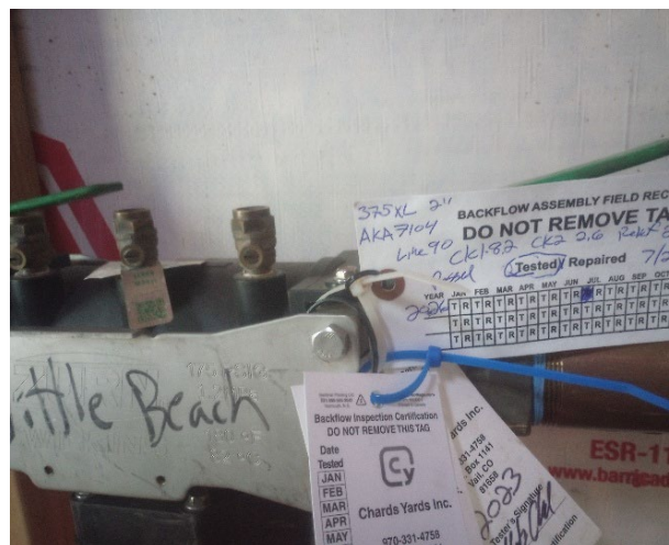
Little Beach Park Backflow Testing
