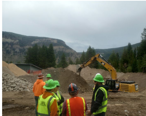
Council WTP Site Visit 7/29
