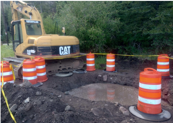
Main Line Water Leak at Maloit Park Rd.
