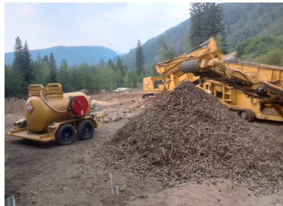
Sediment and Material Screening at WTP
