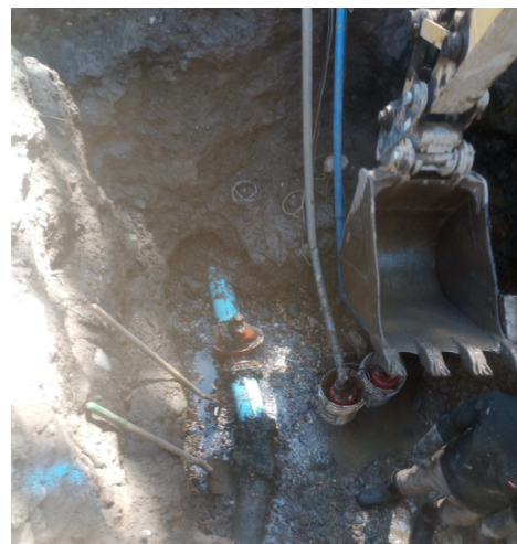
Main Line Leaking Valve
