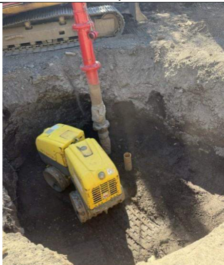
Soil compaction in fire hydrant excavation area.
