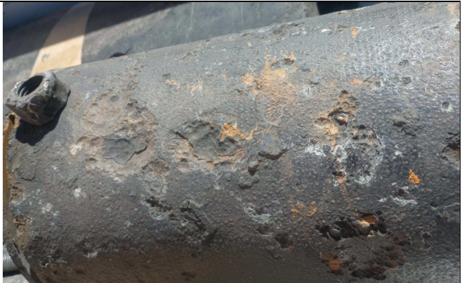
Removed water main pipe showing signs of exterior corrosion.
