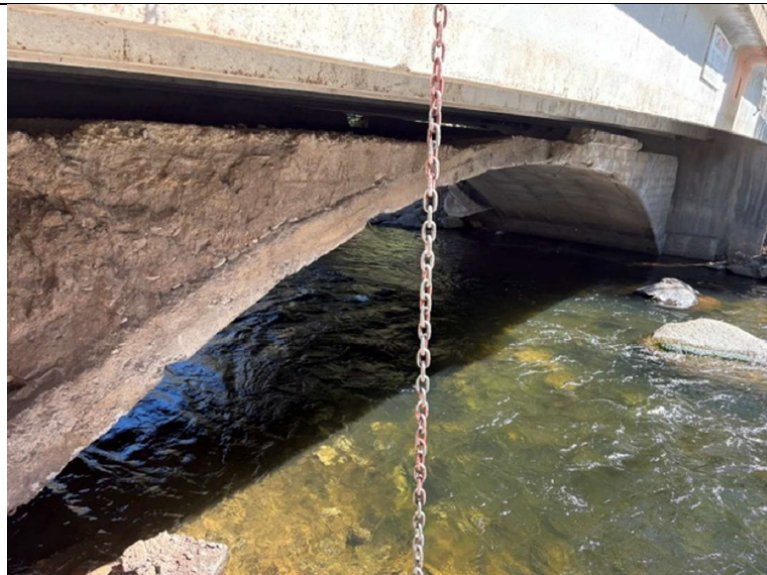
Accumulated dirt on top of the concrete arch.
