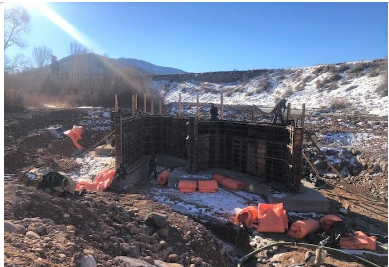
Coffer dams used to isolate the new headgate during the concrete pour.
