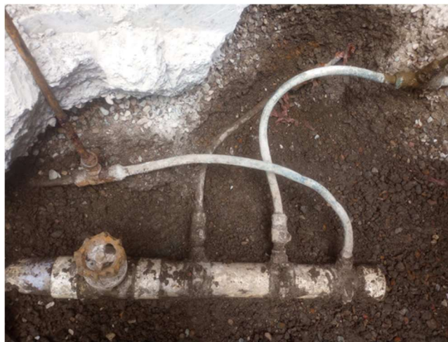
Service connections at 107 Williams Street
