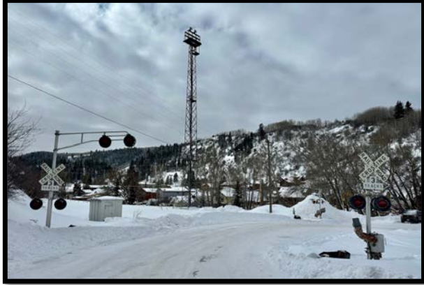
D&RG Railroad Trackside Crossing, Lighting and Signal Equipment
