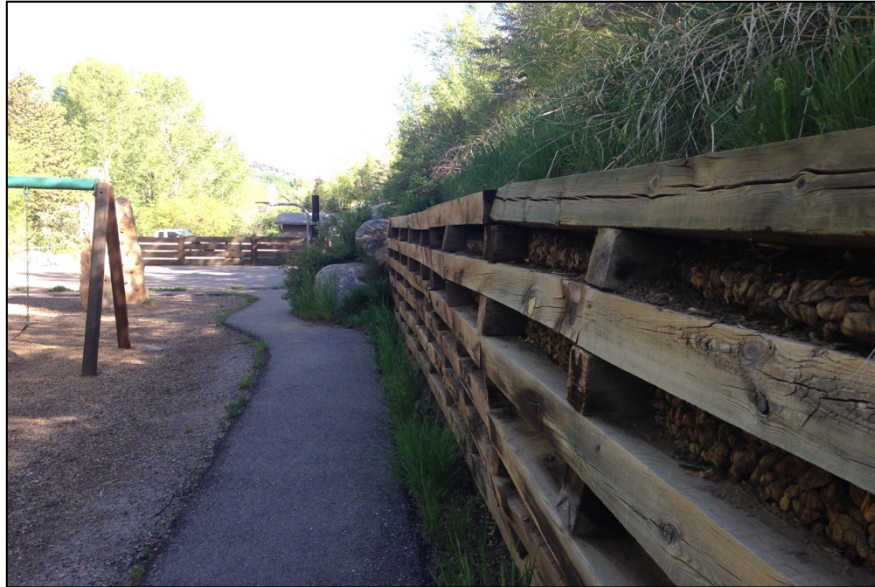
Failing Retaining Wall
